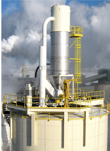
Silo deck equipment support platform with filter receiver, fan, bin vent & jib crane
