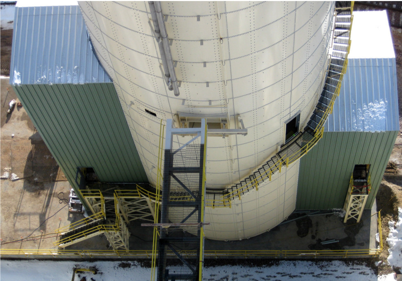
Dog house enclosures with stair access
