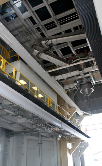
Articulating spout positioner with dust collection, retractable spout and control room
